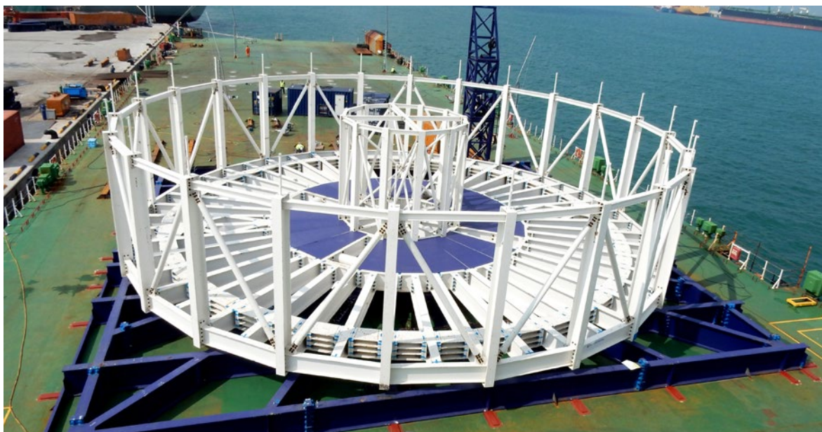
RentOcean's 4000T Turntable being built up at LS Cable quayside in South Korea
