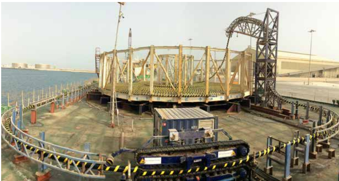
4000T demountable turntable spooling cable in Qatar
