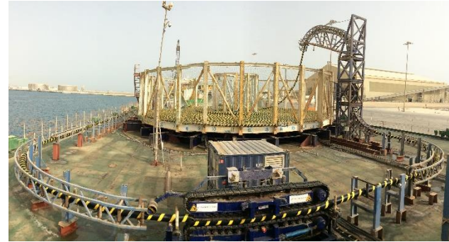
4000T demountable turntable spooling cable in Qatar
