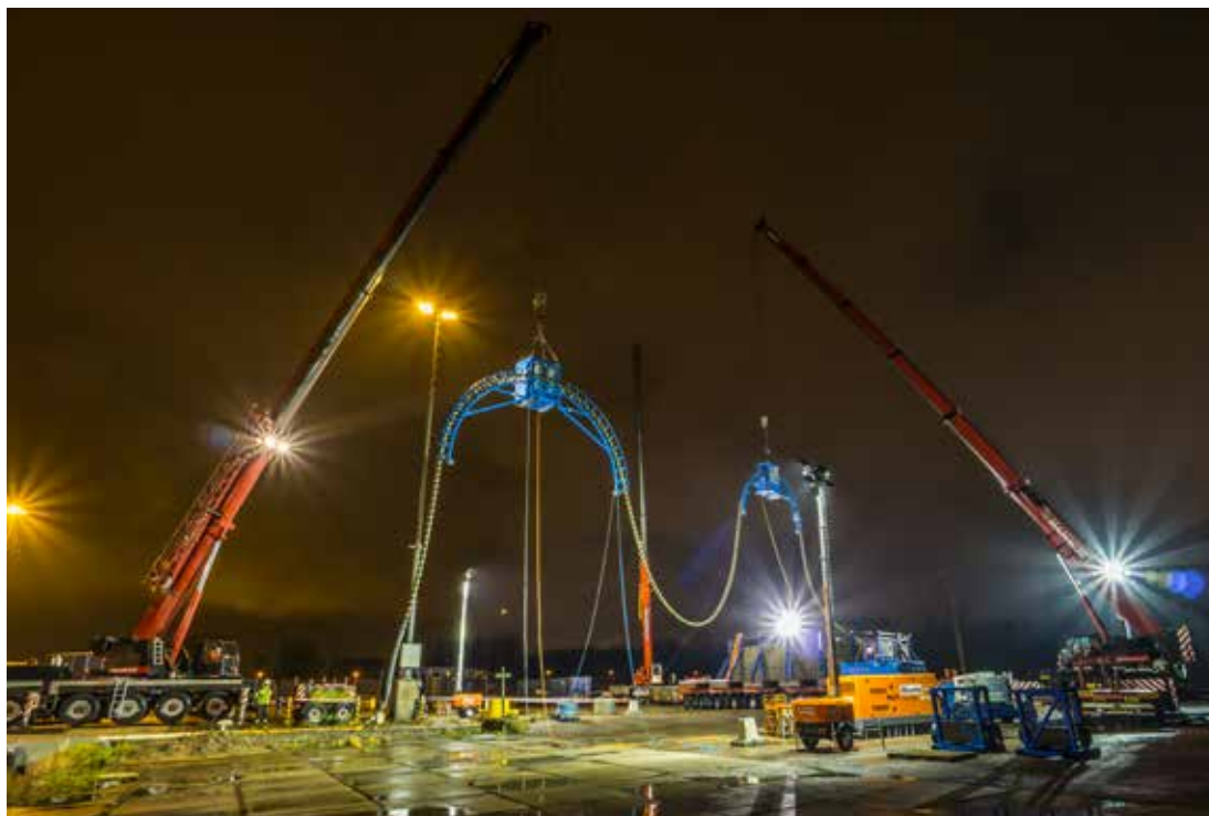
One of the cable loadouts executed at Oceanteam Solutions' storage facility in Velsen Noord.
